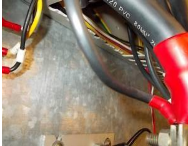
Figure 28: Front 80 mm / 2; rear 10 mm / 2. Unsafe we close the 10 mm / 2 directly to a backup. WU_232_220
