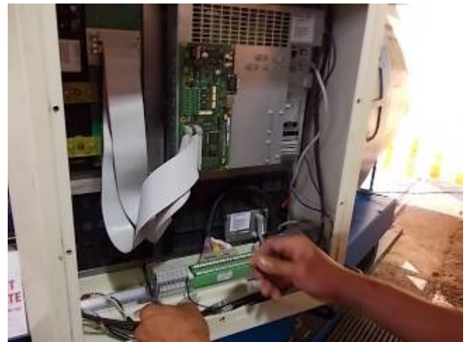
Figure 35: Significant reduction in cables that hang around there. Sure, only about 30%. WU_232_290
