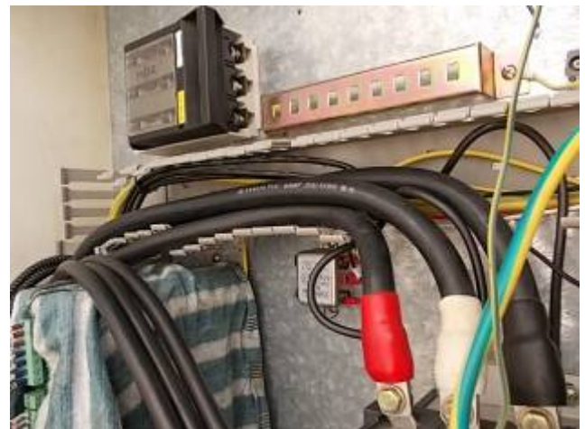
Figure 27: The security system is improved. No wires without protection. WU_232_210
