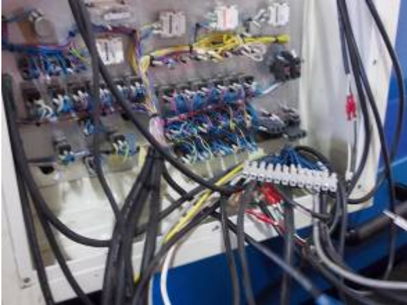
Figure 4: Here is the inside view from the old panel. It is striking that the CNC is connected to a 50-pin cable. We will replace it with a 2-pole Profibus cable. WU_232_40
