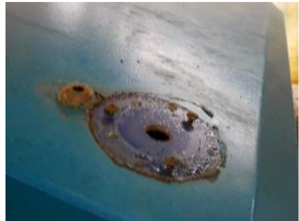
Figure 1: Here was a lamp. Above, where the screw is, there was a hole through which at leaking roof by a storm, the CNC control Fanuc was 18 i destroyed.
