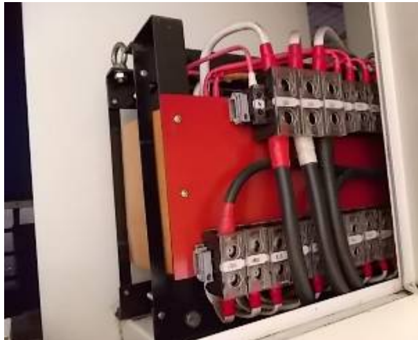
Figure 29: A large transformer, which reduces the 230/400 volts to 115/220 volts. WU_232_230
