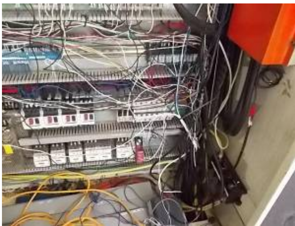
Figure 9: Mixed cable networking. It is striking the machine manufacturer has the 0 conductor and the supply with various colors wired for 220 volts. Cables that were too short were extended in the
