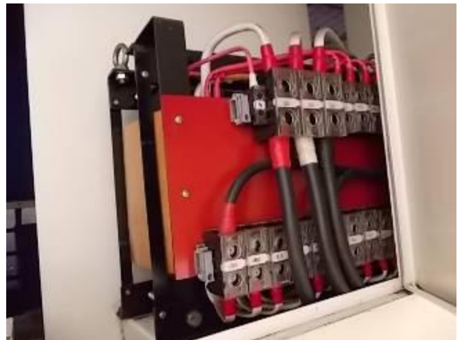
P23) A large transformer which reduces the 230/400 volts to 115/220 volts.
