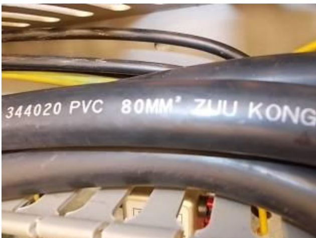
P20) Since there are cables with 80 mm / 2. Since the engine is operated in the country of origin 115/220 volts, this thick cables have been installed.
