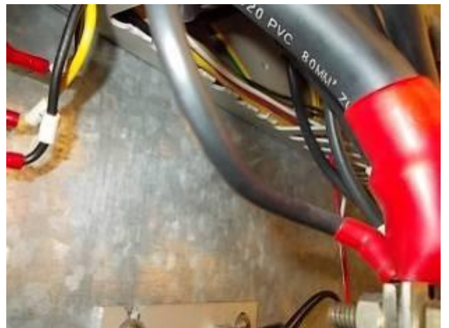
P22) Front 80 mm / 2, rear 10 mm / 2. Unsure we close the 10 mm / 2 directly to a fuse.
