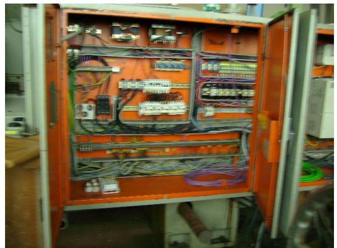
Figure 9: The electrical cabinet much of the old was cleared and new installed.
