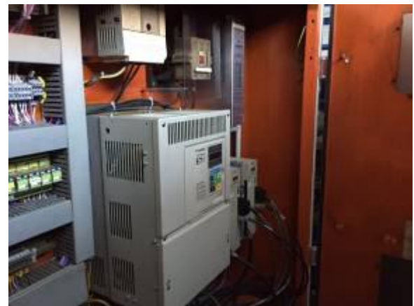
Figure 3: Omron spindle drive 30 KW and Omron feed drives 2 x 3 KW; 20 Nm torque motor. Machine was rebuilt by WIAP AG with new CNC, screw drive and feed motors.
