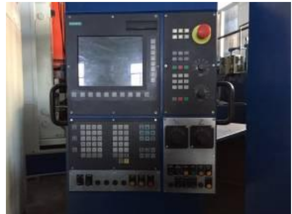
Figure 2: CNC Sinumerik 802 DSL with Profibus system, ADI 4 modules, etc.
