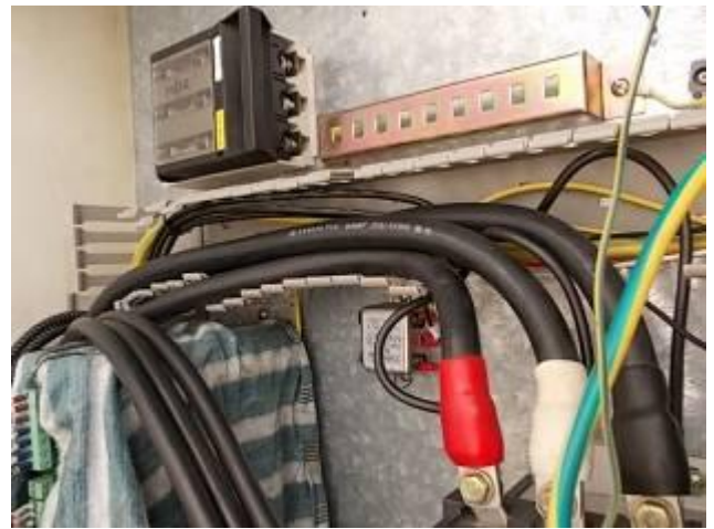
P21) Here we make the security system underst, more safeguards. No thin and thick wires without protection.
