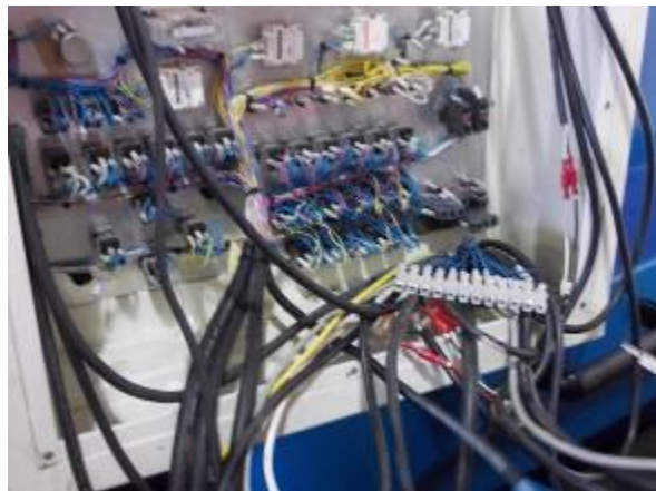
P4) Interior of the old panel. It is remarkable that here a 50-pin cable connects to the front CNC CNC rear. We will replace this with a Profibus cable, 2-pole.
